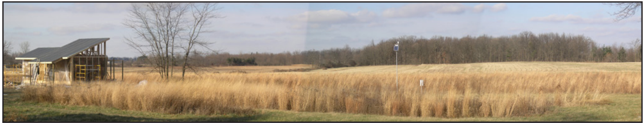
Figure 1 : Eco-Center under construction sited at the south end of a restored prairie, Muncie, Indiana
