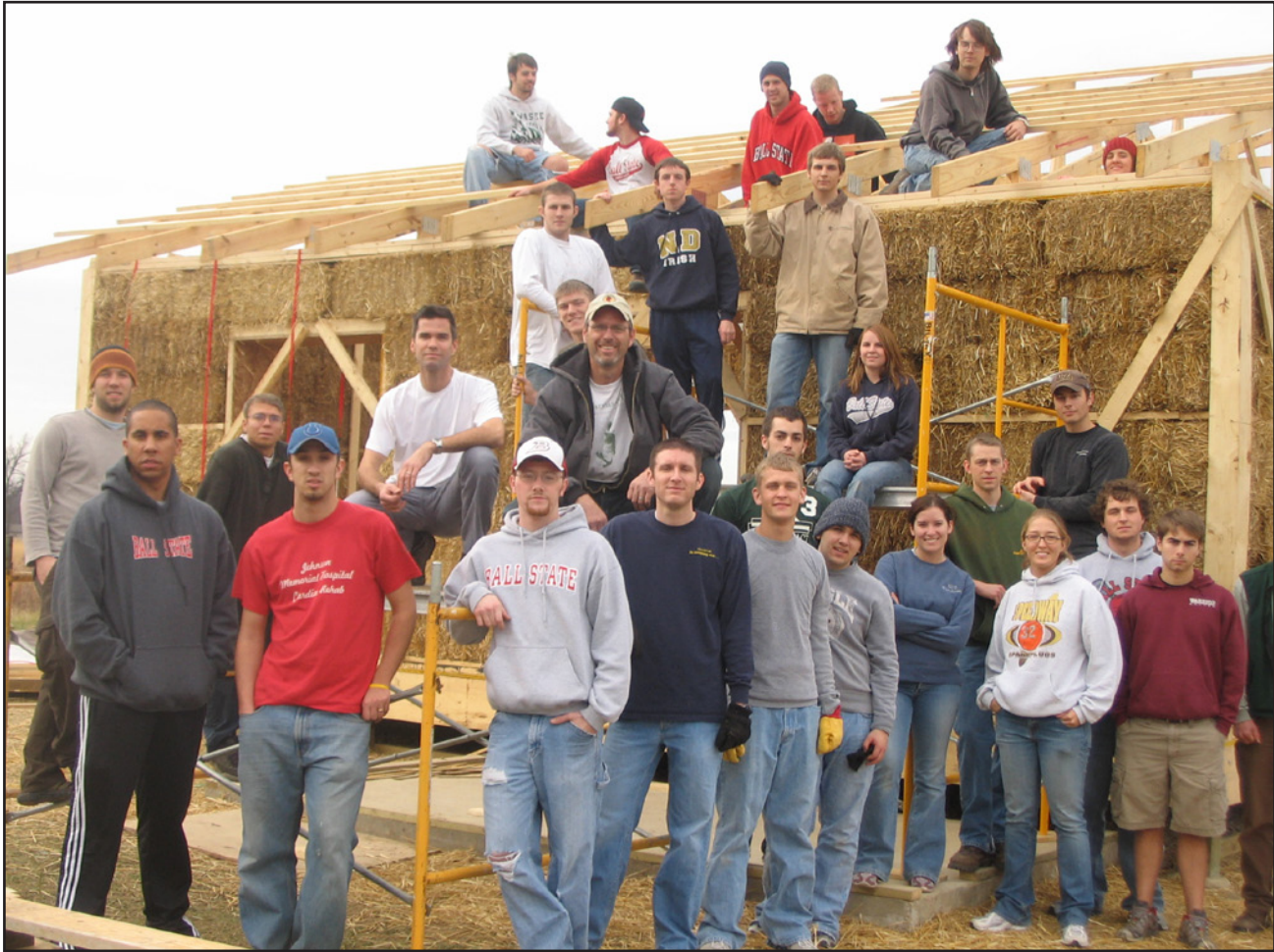
Fig. 3: A proud moment after the bales trusses were “raised” onto the bale wall
