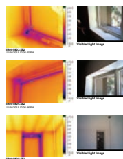
Thermal Imaging and Testing of Installed Components
